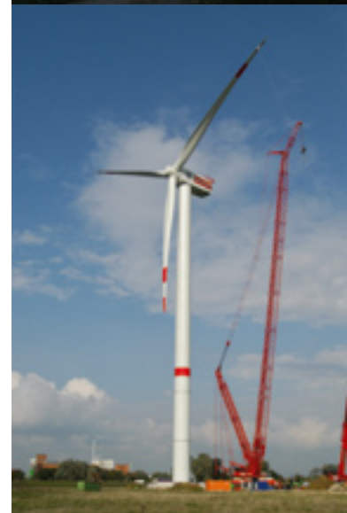
New generation of 2004: Based on Bonus technology Siemens installed its prototype with a 3.6 MW turbine in Høvsøre, Denmark (on the top). The prototype of Repower 5M with a 5 MW turbine was built up in Brunsbüttel, northern Germany (in the middle).
