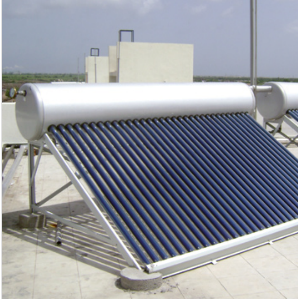
The Indian supplier Kotak Urja is one of the few companies which supply both systems with flat plate and vacuum tube collectors.
