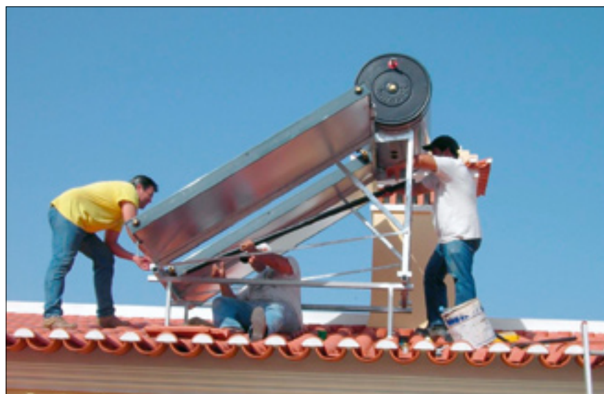
Three handymen installing a system with two collectors in Portugal. Ouraset (Turkey) puts the tank in the middle.
