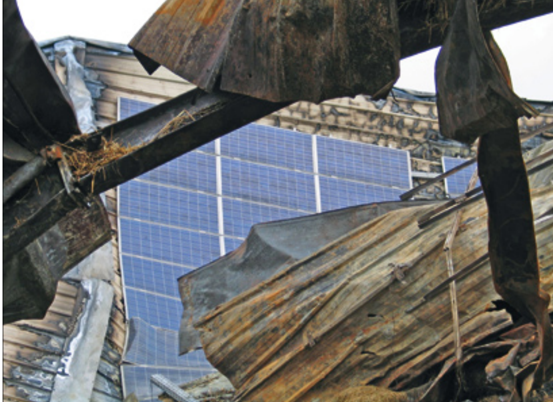
Up in smoke: Fire damage is rare, and usually PV systems cannot be repaired afterwards.
